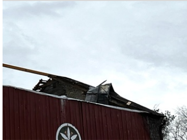
The work began in September 2022 with the removal of the existing leaking roof and badly damaged purlins.
